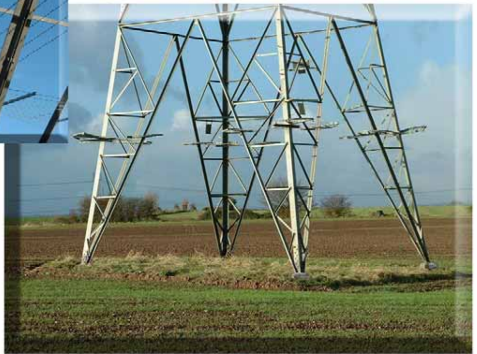
275kV AND 400kV NGC TOWER ACD's
